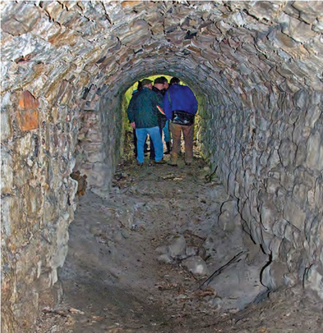
The adit has collapsed behind the photographer
